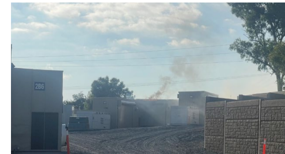
Terra-Gen battery storage facility caught fire
