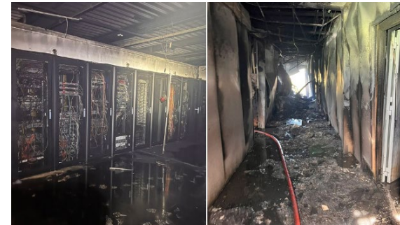
Data center fire in France
