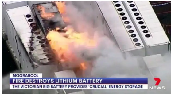
Tesla Megapack on fire at Victorian Big Battery, Australia
